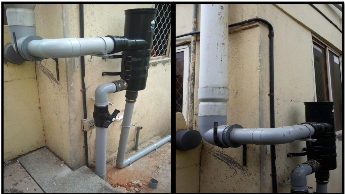
Rain Water harvesting structure to recharge the bore well
